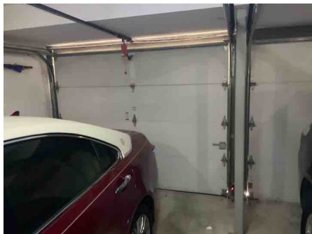
Unprotected garage door
