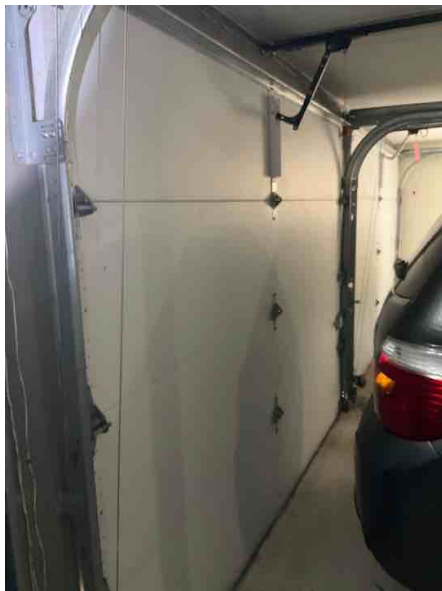
Unprotected garage doors
