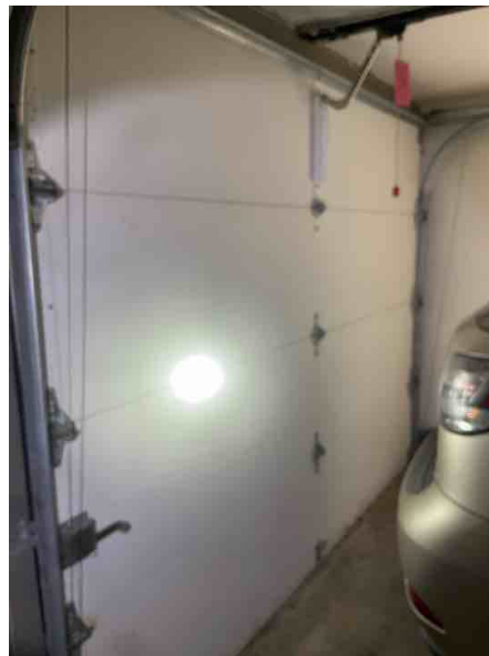
Unprotected garage door
